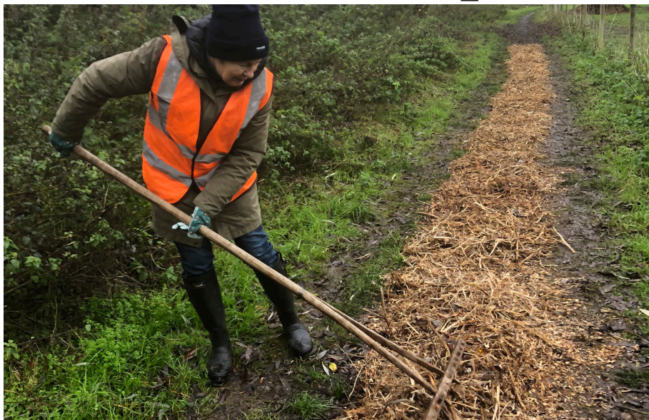
Wood chip spreading along a path by the side of the River Lark.
