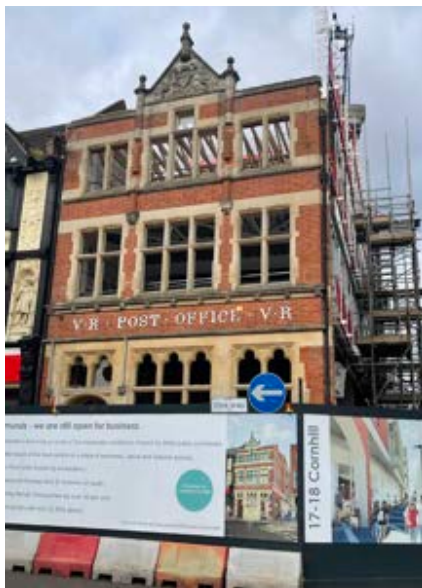
The front of the former Post Office in Cornhill with trusses and steel beams removed prior to scaffolding being erected to allow for conservation work.
